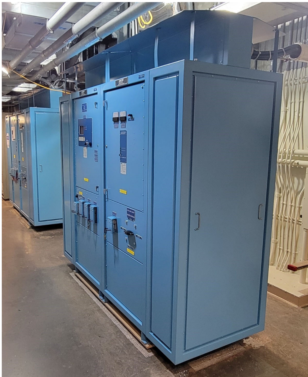
Figure 1 – First Safety-Related NDPP Digital UPS at Hope Creek Station
