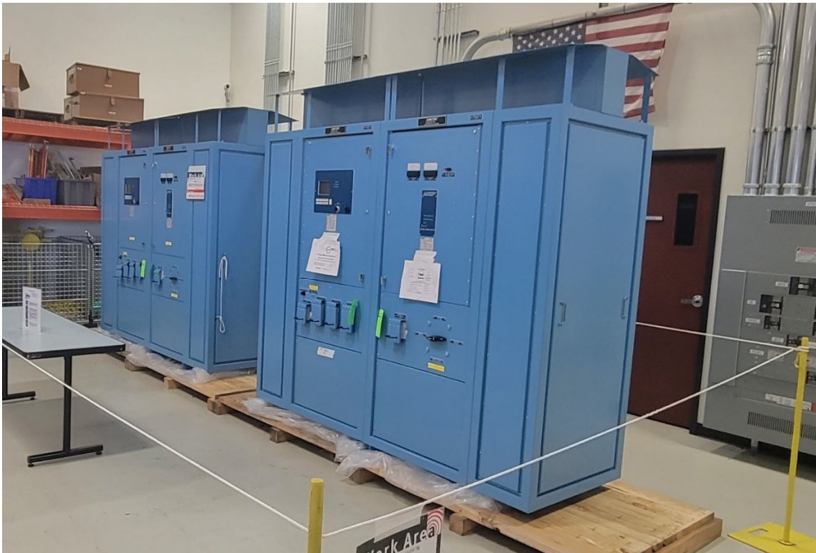
Figure 3 – Inverter Test Lab Used for Pre-Testing and Acceptance Testing
